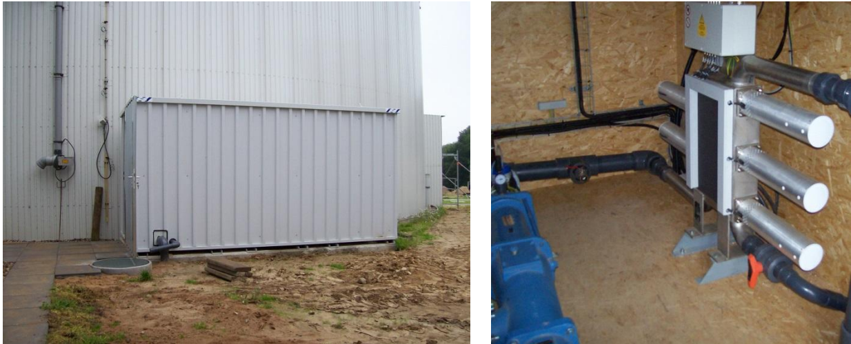
Figure 1: Container with system from the outside and inside (US module and pump are shown)
